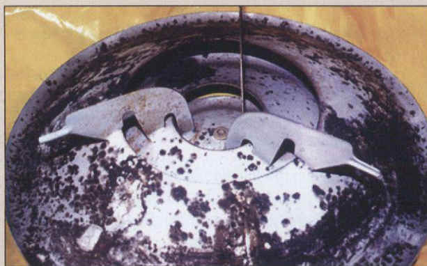
Mold spores may become airborne through a building's HVAC system, as is evident in the air diffuser above.
