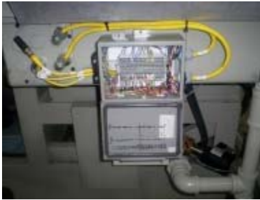
Door switch wiring box, terminal strip, and wiring.
